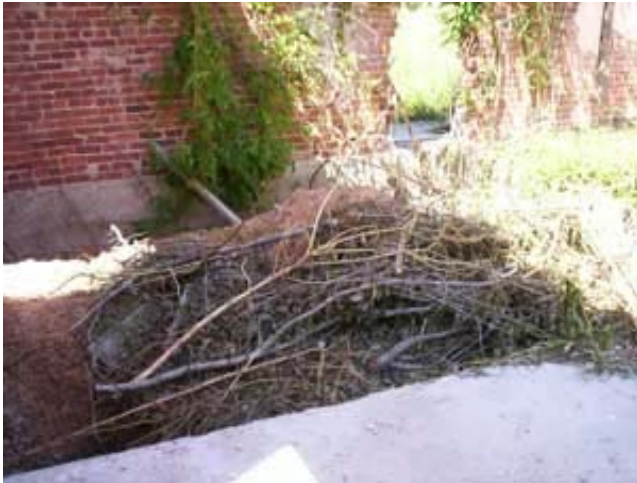
The hole in the Coppedge Building floor that once served as a storm cellar has now been filled with dirt and branches.
